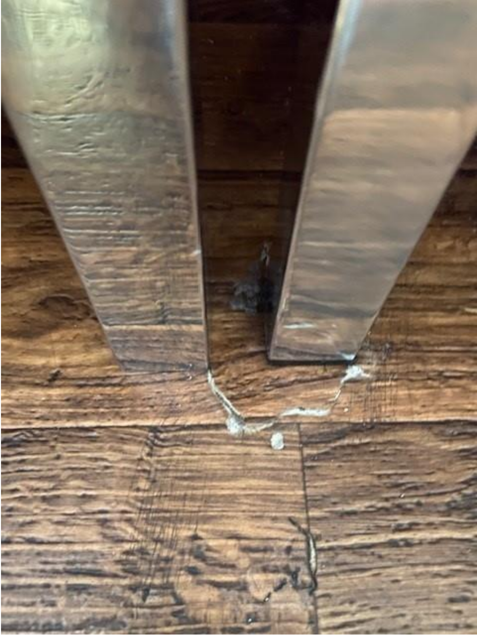
Pictures of the damaged flooring at Horizon Home February 9, 2024
